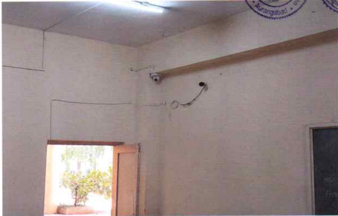
Camera in Hall No. 3
