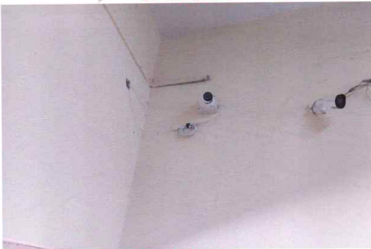
Camera in Hall No. 2
