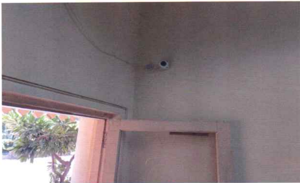
Camera in Hall No. 4
