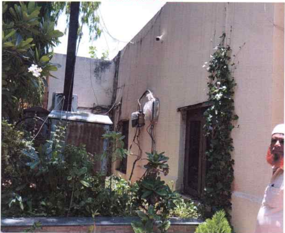
Camera near entrance
