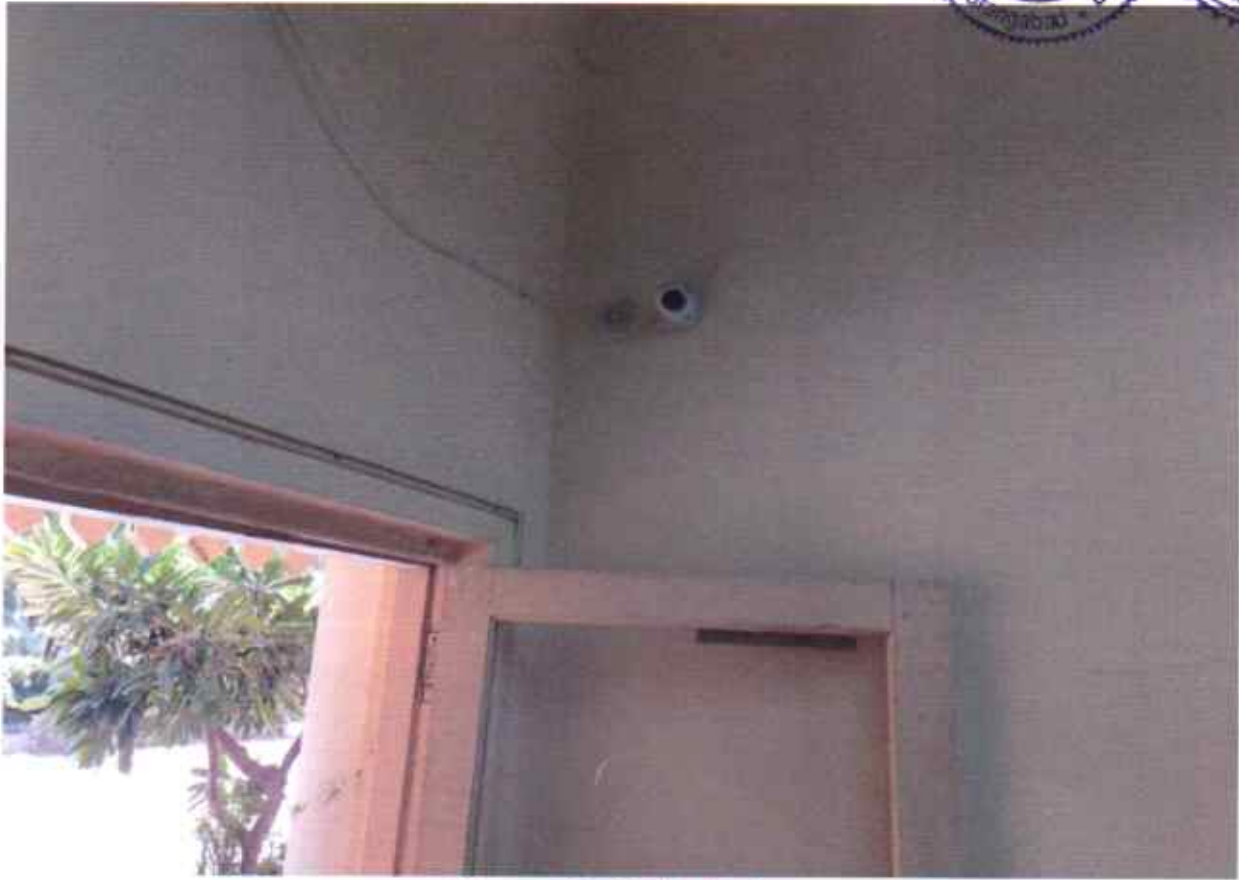
Camera in Hall No. 5
