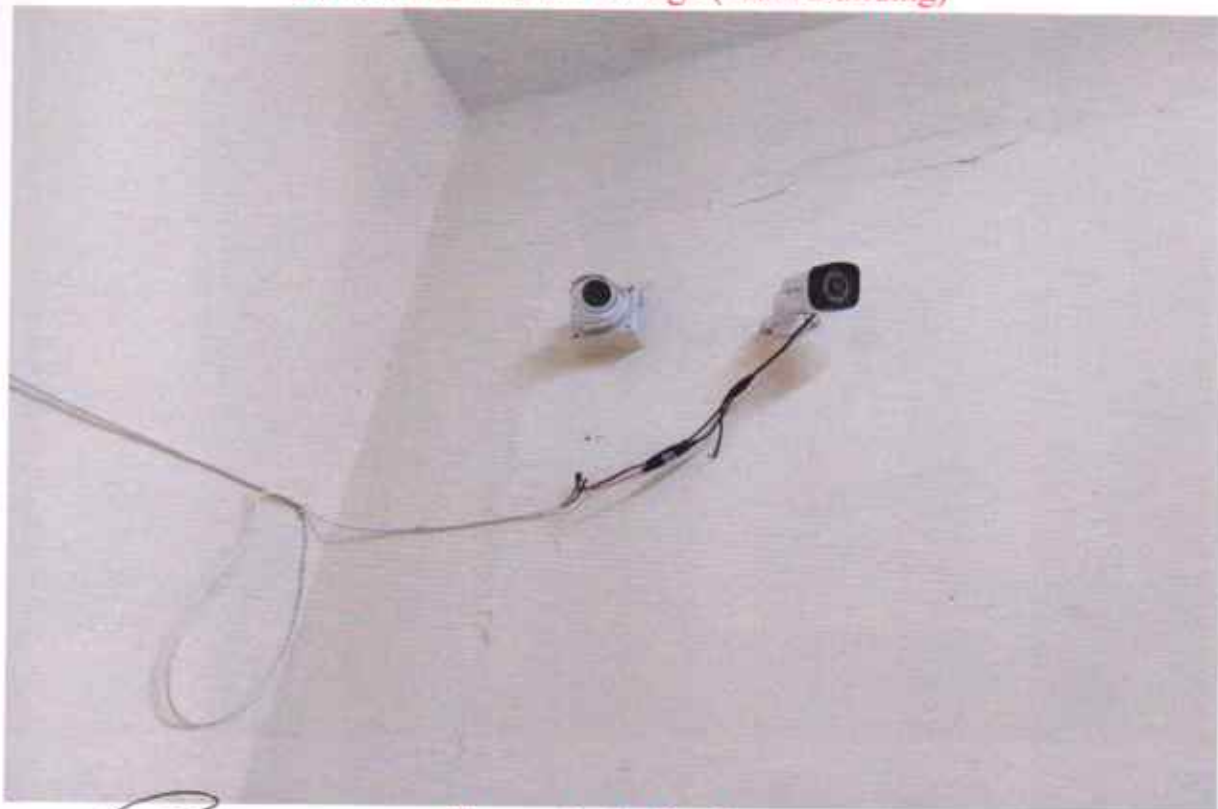
Camera in Auditorium
